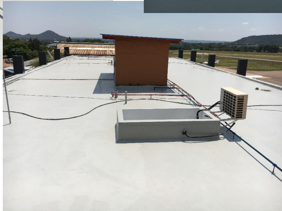
Figure 8: Overview of the upper west-section showing the coating system,
