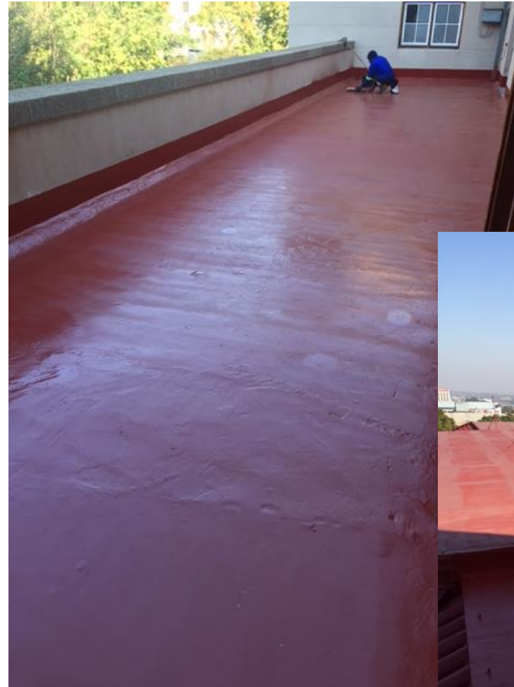
Figure 1: An area of the roof with a concrete substrate after application of the coating/waterproofing system
