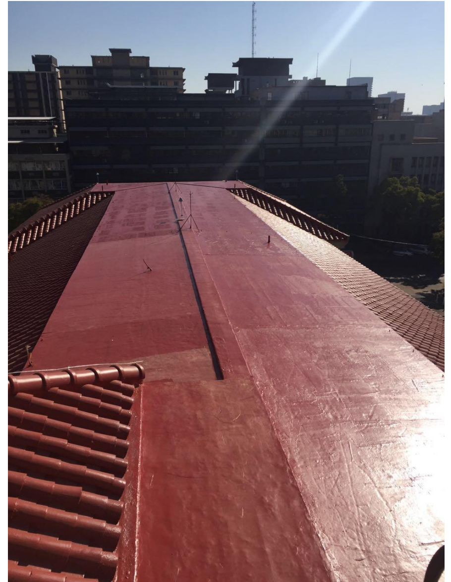
Figure 5: The area of the roof with cementitious polymer on Polystyrene boards after application of the coating/waterproofing system
