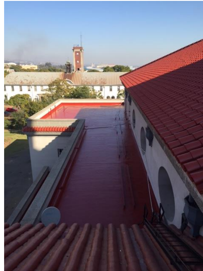
Figure 3: The area of the roof with clay tiles and concrete substrate with bitumen after application of the coating/waterproofing systems
